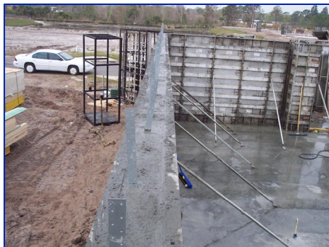
A cast-in-place concrete wall just after pouring and placement of truss tie-down embeds.
